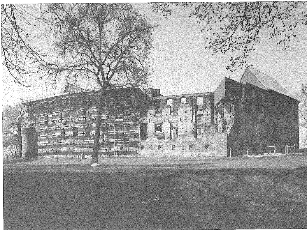
FIG. 8. A view of the castle from the south-east during restoration. The work is being carried out in stages simultaneously from west and east, and the large aperture in the south-east corner has been closed. The roof construction incorporates a horizontal steel truss which connects the east and west wings, simultaneously fixing the load-bearing columns and stabilizing the ruined walls.
