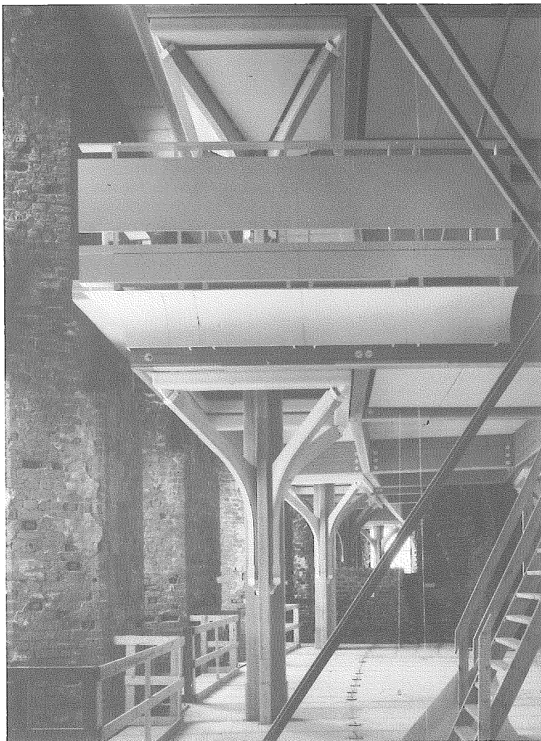
FIG. 11. The interior of the south wing. The new load-bearing structures have been erected; the laminated timber columns with their 'branches' continue through the storey partitions and terminate with a white pyramidal capital. The protective railings, struts and stairs seen here are temporary. ( Photograph: Ernst Kallesoe )
